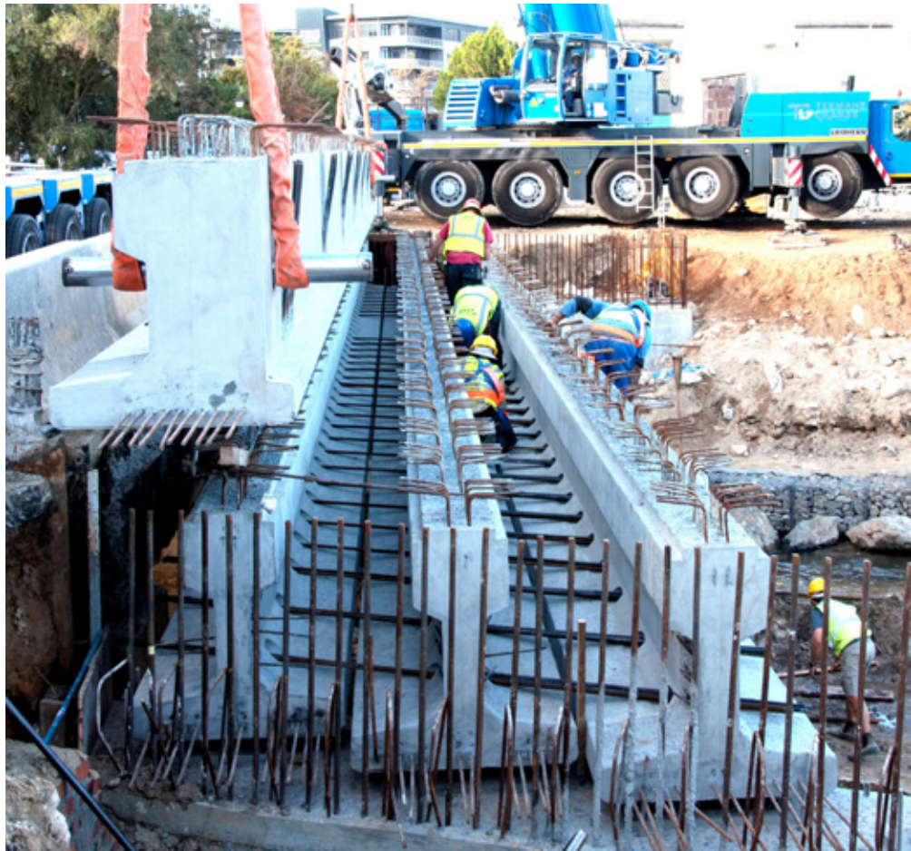
Workers insert rebar through sleeves situated in the beams' lower web sections
