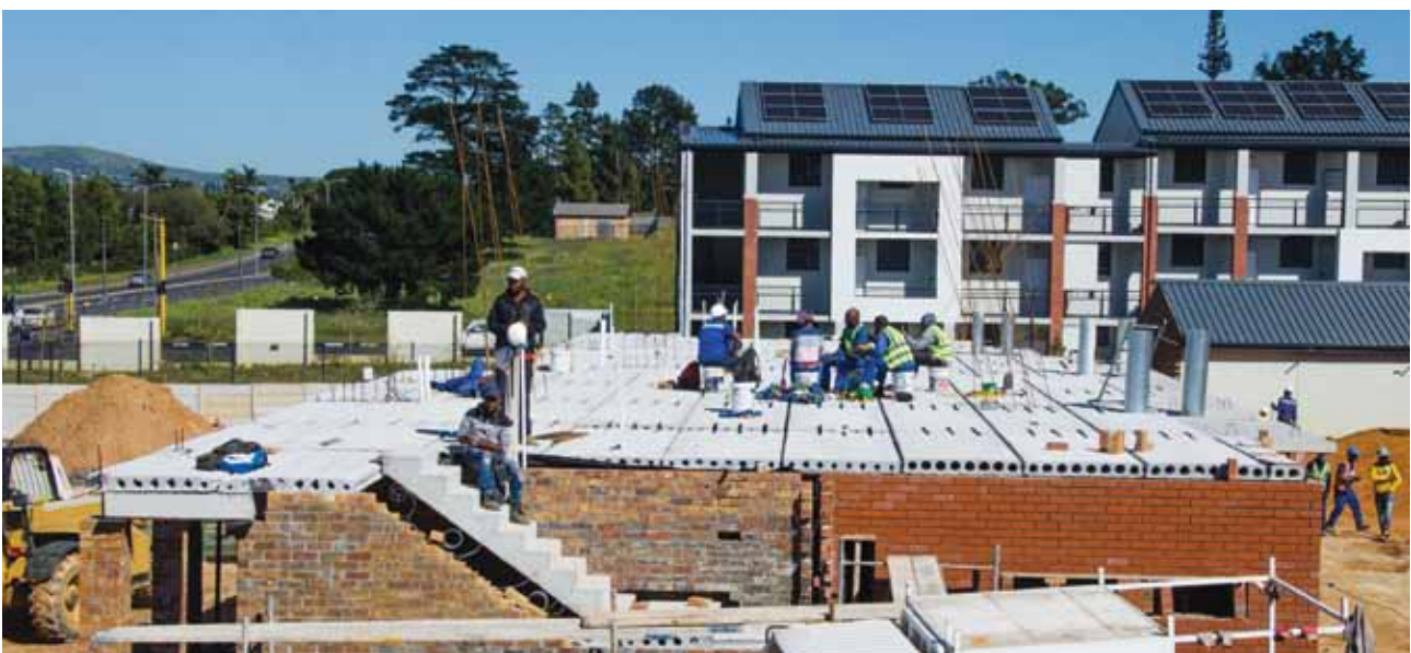
An apartment block under construction showing a precast concrete staircase and the first-floor hollow-core slab flooring.
